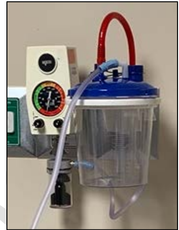
Figure 3 Typical healthcare facility wall suction.
