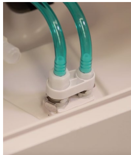
Figure 33: HPM Gas Lines Connections
