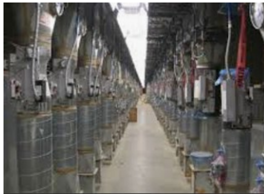
Figure 69 – State-of-the-Art White Oak Infrastructure: Advanced Air Terminal Units Supporting Laboratories
