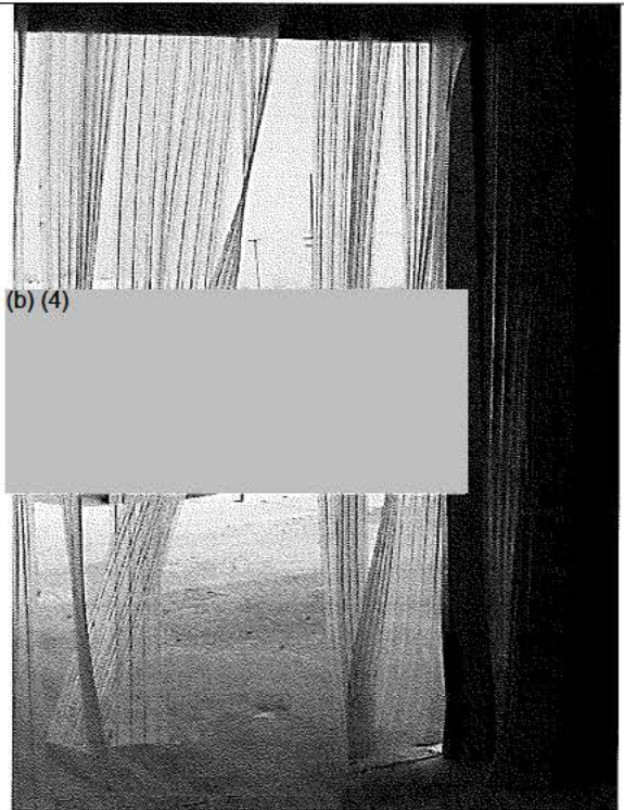
Obs. 1.a. Digital Photo 1572 – Plastic strip door curtain located at the north production warehouse dock door was missing a strip. Raw product is stored approximately 20 feet from the plastic strip door curtain.
