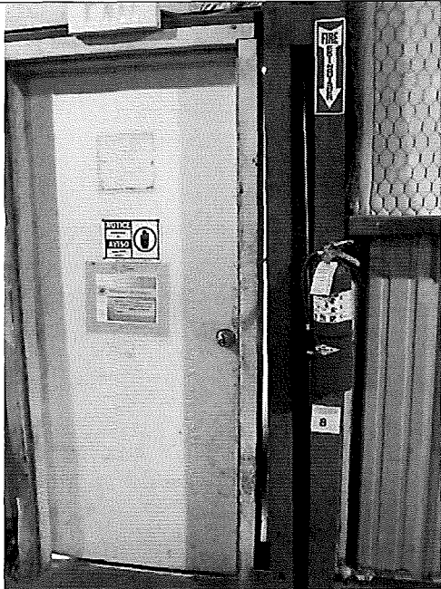
Obs. 1.b. Digital Photo 1529 – A gap approximately 1/4 inch wide by 7 feet high, was observed along the northern side of the door frame.
