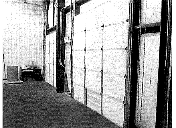
Obs. 1.c. Digital Photo 1565 – Gaps were observed on the south dock door in the peanut butter cleaning room, and located approximately 12 feet from raw product.
